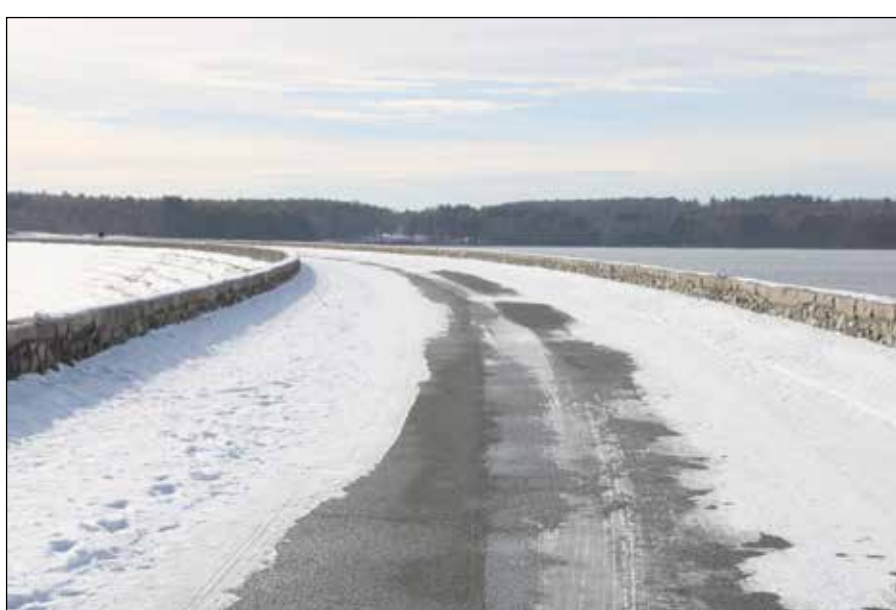
A roadway passes over the top of Winsor Dam. Although it is no longer open to public vehicles, walkers and bicyclists are welcome to explore the massive structure.
